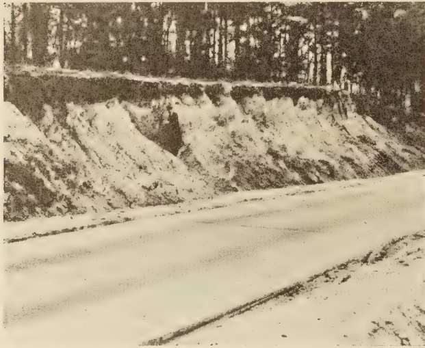
FIGURE 2.—EROSION OF BACK SLOPES IS VERY IRREGULAR AND THERE IS CONSIDERABLE SLOUGHING OF MATERIAL INTO DITCHES
